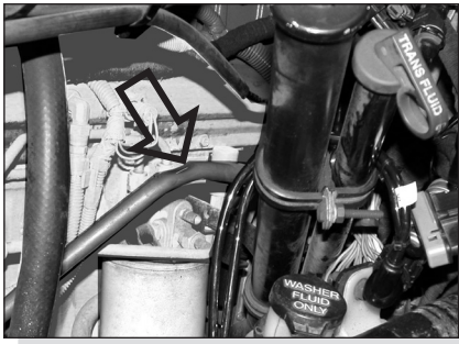
Damaged discharge line shown.
