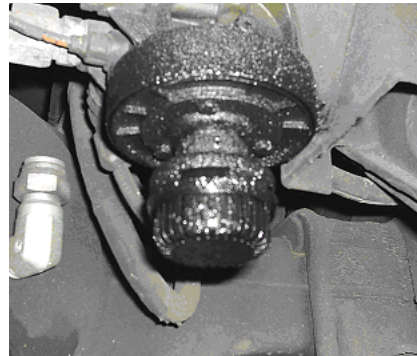
Air dryer exhaust with oil present
